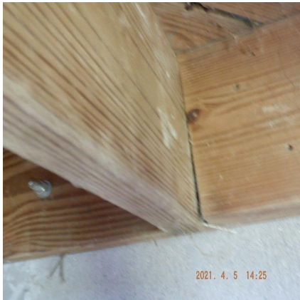
DECKS / BALCONY: No Mechanical Joist Hangers - Upper Deck
