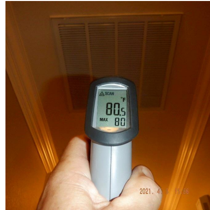
Cooling: Return Air Temp
