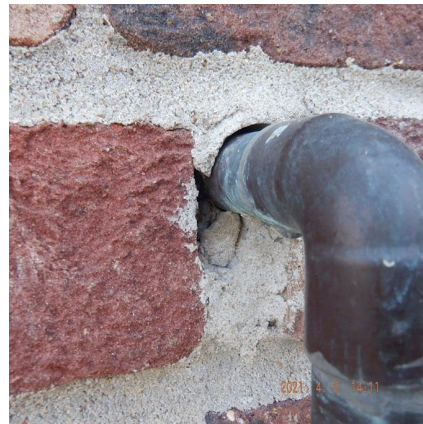
EXTERIOR SURFACE: TPR Plumbing Opening Into Home
