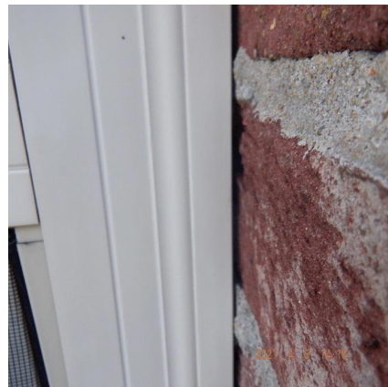
WINDOWS: No Caulk on Exterior Windows
