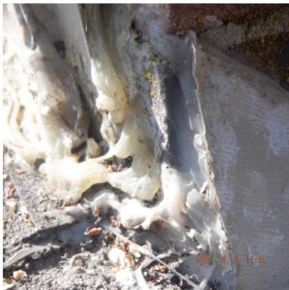
FLASHING/VALLEYS: Deterioration Caulk
