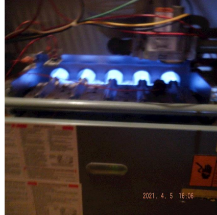
Heating: Furnace Burners Operational
