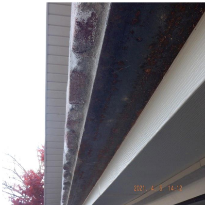
EXTERIOR DOORS: Unpainted Lintel
