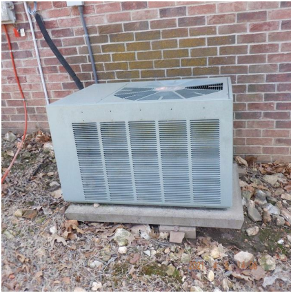
COOLING: A/C Unit - Date of Mfg 11/2003
