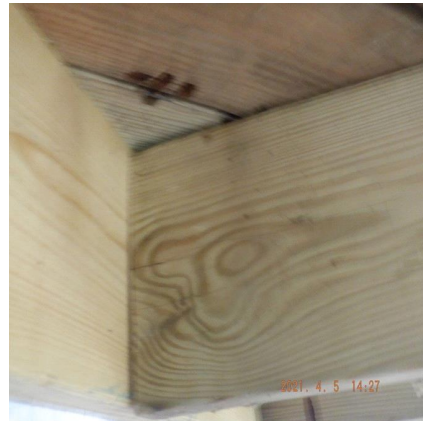
DECKS / BALCONY: No Mechanical Joist Hangers - Lower Deck
