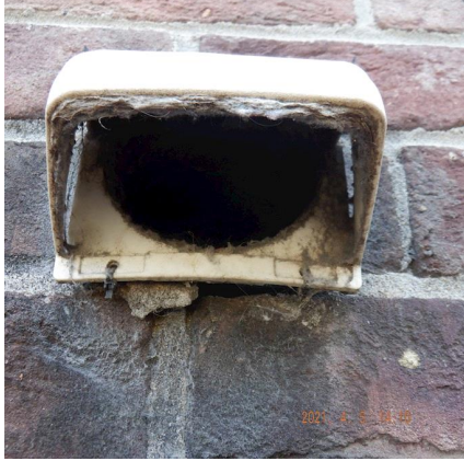
EXTERIOR SURFACE: Broken Dry Vent Cover - Missing Flap
