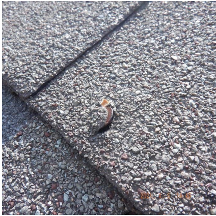
ROOFING: Lifted & Exposed Nail
