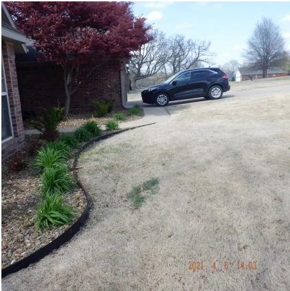
GRADING / DRAINAGE: Negative Slope Southeast Corner
