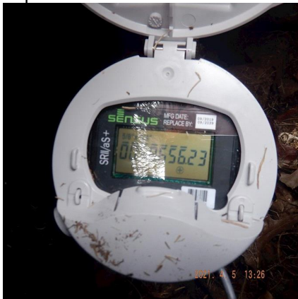
PLUMBING: Initial Meter Reading
