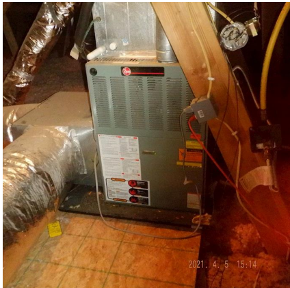
HEATING: Furnace In Attic - Date Of Mfg 10/2003
