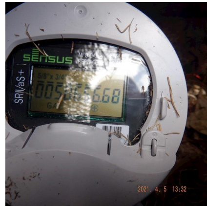
PLUMBING: Meter Reading 6 Minutes Later - Leak Detected - Master Toilet
