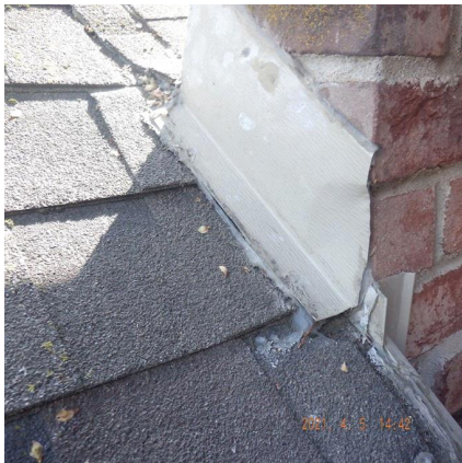
FLASHING/VALLEYS: Caulk Around Flashing Lifted & Deteriorating
