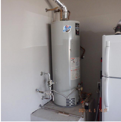
Water Heater: Gas Hot Water Heater - Date Of Mfg 7/2003
