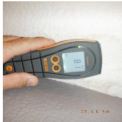
GUEST BEDROOMS (3): Water Damage Spot In Ceiling
