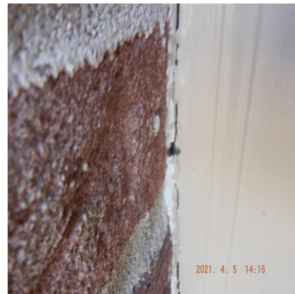
EXTERIOR DOORS: Cracked Caulk Between Brick & Door Frame
