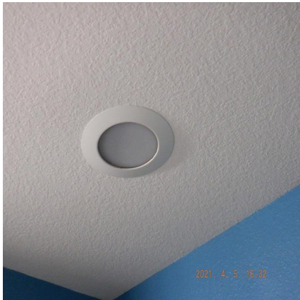
MASTER BATHROOM: Light Out Over Shower
