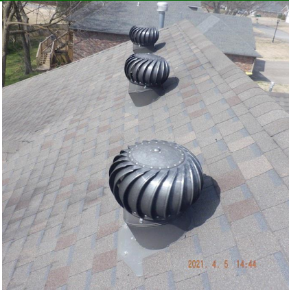
Attic Ventilation: Turbine Vents
