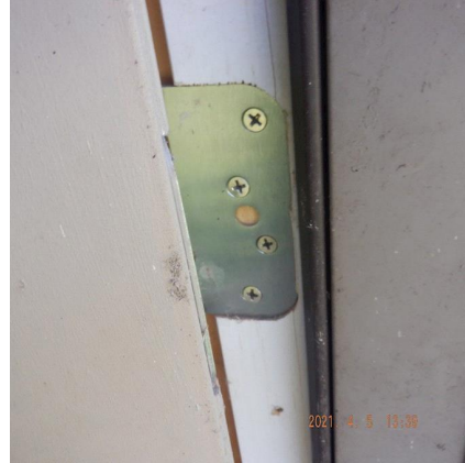
EXTERIOR STRUCTURES - SHOP: Missing Long Screws
