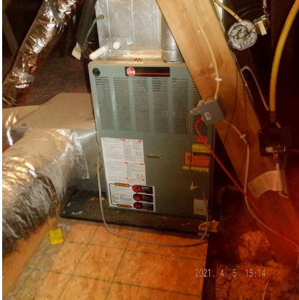
Heating: Furnace In Attic - Date Of Mfg 10/2003
