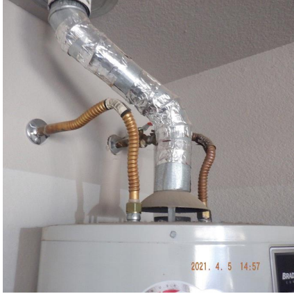
WATER HEATER: No Expansion Tank
