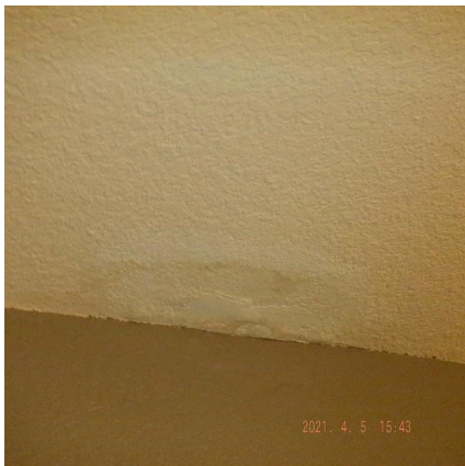
GUEST BEDROOMS (3): Water Damage Spot In Ceiling
