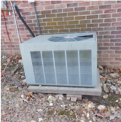
Cooling: A/C Unit - Date of Mfg 11/2003
