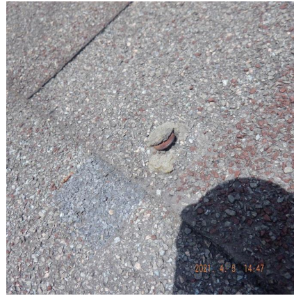
ROOFING: Lifted & Exposed Nail
