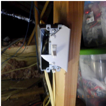
ATTIC ELECTRICAL: Broken Cover On Light Switch
