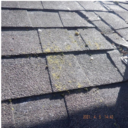
ROOFING: Moss On Roof
