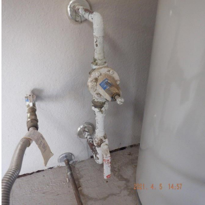
Plumbing: Main Water Shut Off
