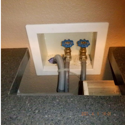
Laundry Facilities: Laundry Hook Up
