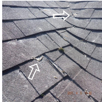
ROOFING: Deteriorating Caulk
