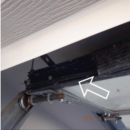
OVERHEAD GARAGE DOORS: Missing Weather Strip
