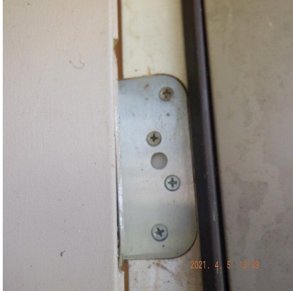
EXTERIOR STRUCTURES - SHOP: Missing Long Screws
