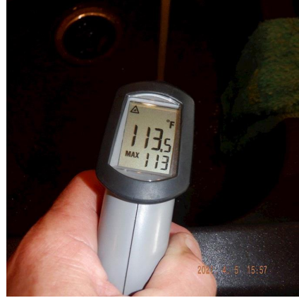
Water Heater: Water Temp at Kitchen Sink
