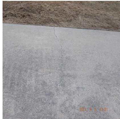
Driveway: Minor Cracks
