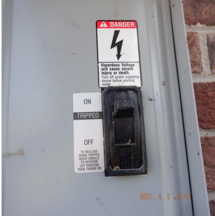
Electrical: Main Electrical Shut Off
