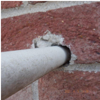
EXTERIOR SURFACE: Condensate Plumbing Opening Into Home
