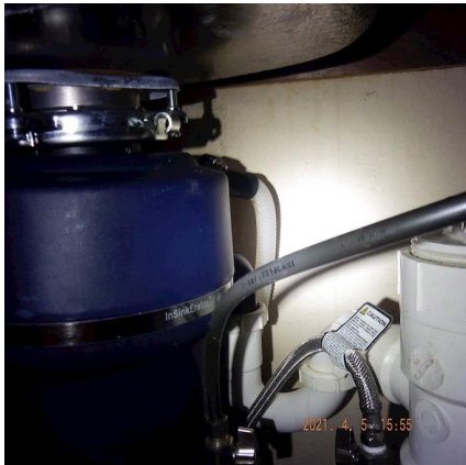
KITCHEN: Improper Dishwasher Cross-Flow
