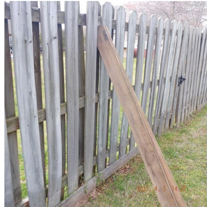
FENCES / GATES: Broken Fence Posts
