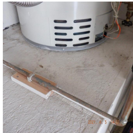
WATER HEATER: No Drain Pan or Drain Line
