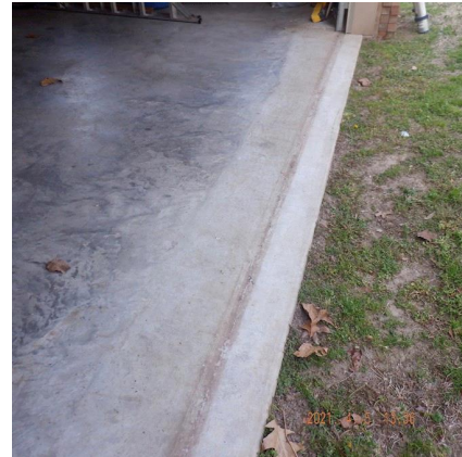
EXTERIOR STRUCTURES - SHOP: Negative Slope Into Shop
