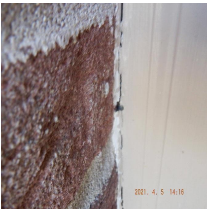
WINDOWS: Cracks in Caulk on Exterior Windows
